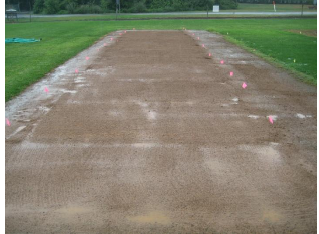
Figure 7. After installation, plots received 0.8 inches of water (combination of irrigation and rainfall)
