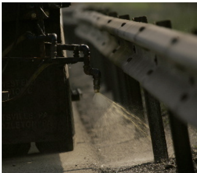
Figure 1. Most total vegetation control applications to roadsides are fixed-pattern, truck-based treatments to guiderails, concrete barriers, and shoulders. Signposts and traffic islands are treated with a handgun application.
