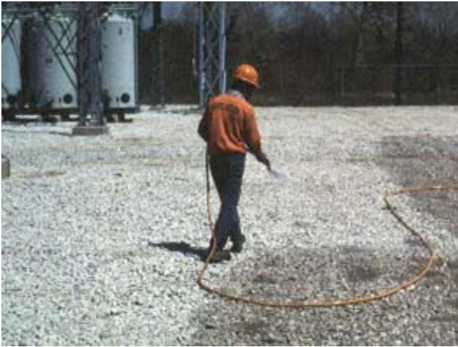
Figure 17. A common industrial site application is made with a sprayer with several hundred feet of hose equipped with a handgun with an off-center spray tip allowing the applicator to treat an 8 to 10 ft swath.
